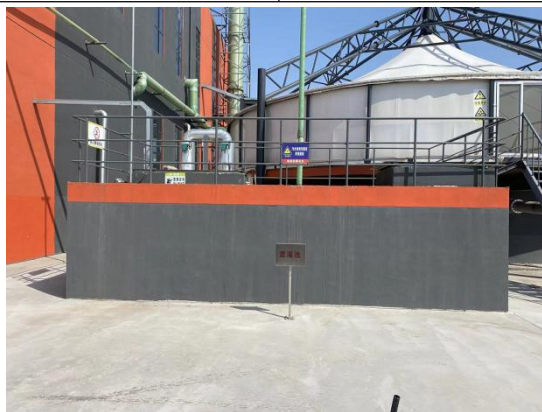
污水站设施—滤液池
