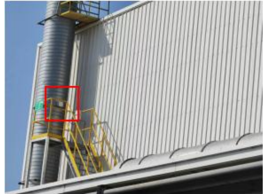
排气筒 DA001 采样口及 Z 字梯
